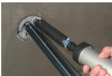
No more leakage
